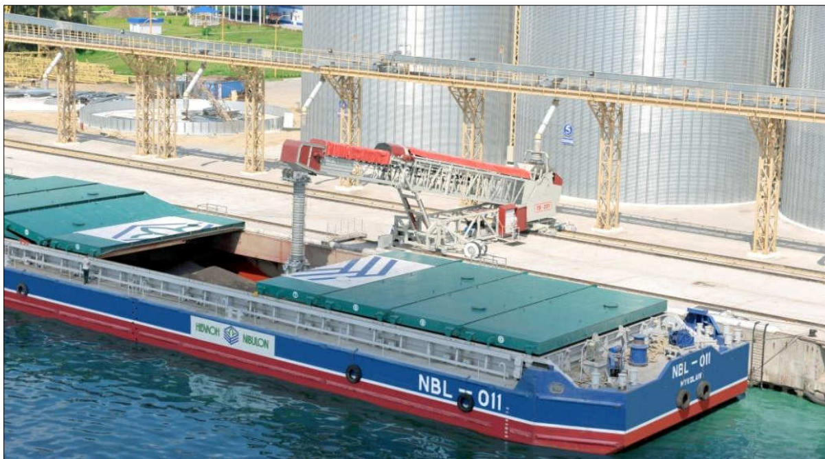
Figure One - TS 227 Rail Mounted Mobile Ship-loader fed directly from Overhead slatted Conveyor to Barge
