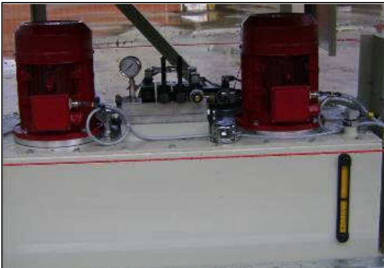
Integrated Electric Hydraulic Power-pack
